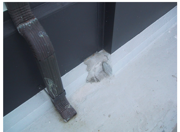
Crumbling concrete at the corners
